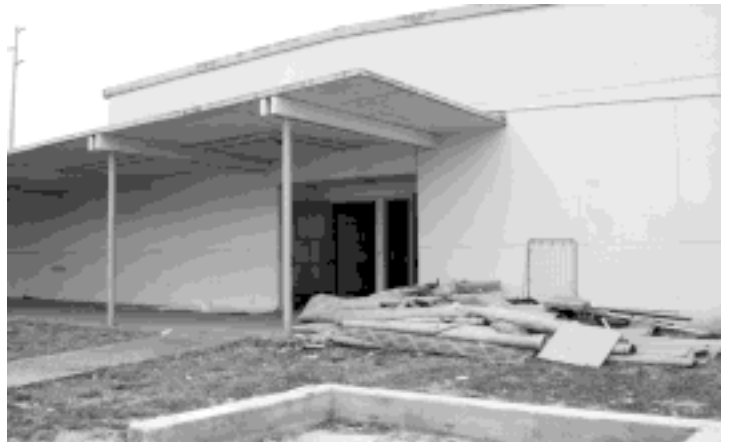
Cleaning out the old carpeting from the Angle Lake School Annex building.
